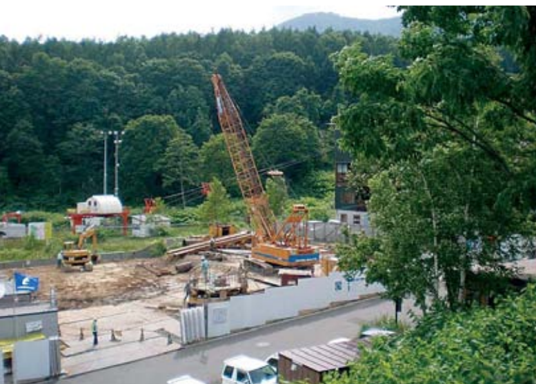
Foundation works commence at the Alpen Ridge site with the ski lift pictured in the background.
