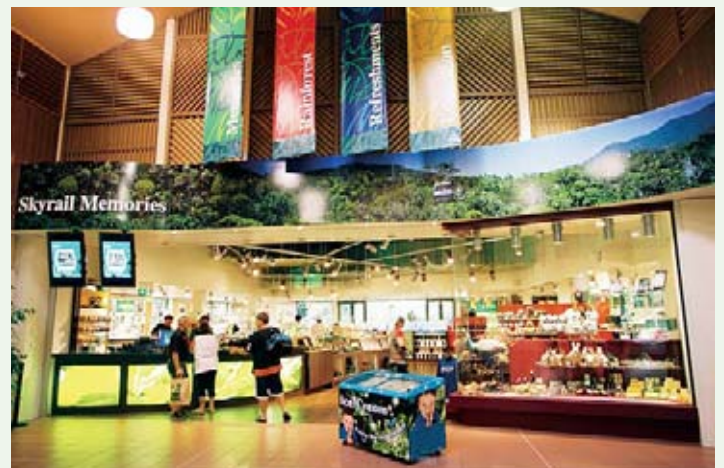
The Cairns Skyrail project combined new and refurbishment works across five separate stages ... cafe and retail; new ticket/sales area; refurbishment of administration area; rail ticket booth; new offices and workshops. The new cafe and retail portion of works is now complete and has been trading since May.
